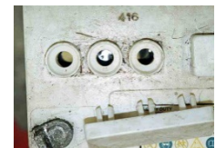
Check battery electrolyte level
