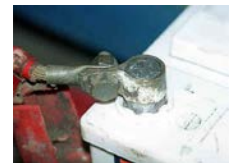
This terminal needs cleaning
