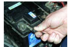
Checking the battery cables for tightness and condition
