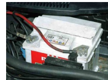
Battery terminals should be...
