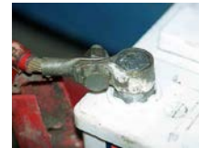
Check terminals for corrosion
